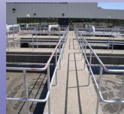
Compressed air bubbles up through the tanks
