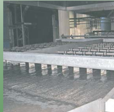
Waste activated sludge is thickened on a gravity belt
