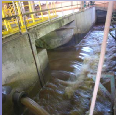
Water pours into the Headworks building
