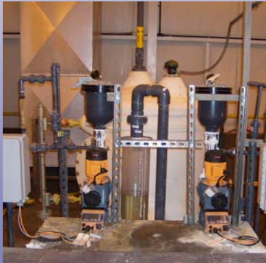
Dechlorination pumps ready the effluent
