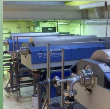
The centrifuges separate water from sludge
